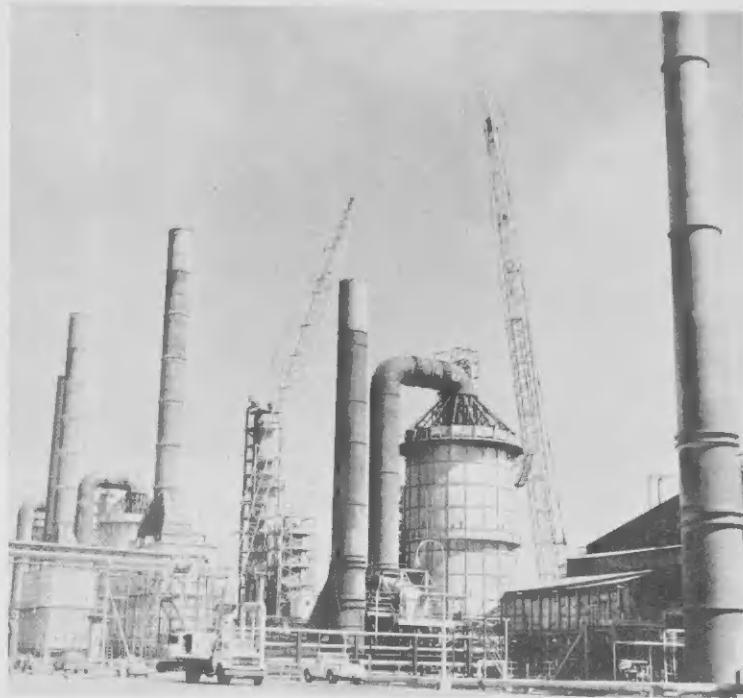
These two cranes are utilized jointly to erect new stack section. Furnace at right, with 150-ft long duct got new insulation lining. E dos gruanan aki ta traha conhuntamente pa instala seccion nobo di e stack. Forno na drechi, cu su coneccion a haya insulation nobo.
